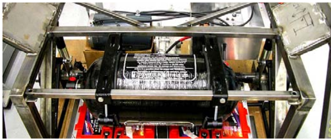
Hydrogen pressurized tank
